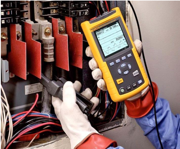
Figure1: Harmonic test of 33/11kv distribution transformer
